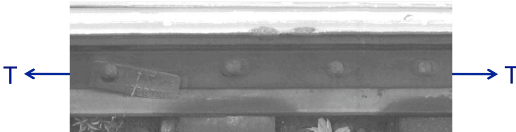
A: Original Image Switch Point Bolts
