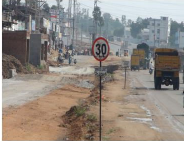
Fig. 11: Dilapidated sign boards require regular maintenance.
