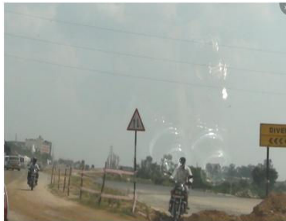
Figure 12: Placement of sign boards is not correct for the traffic playing from Hyderabad to Yadagiri Direction. Further this sign board is missing at most of the locations.
