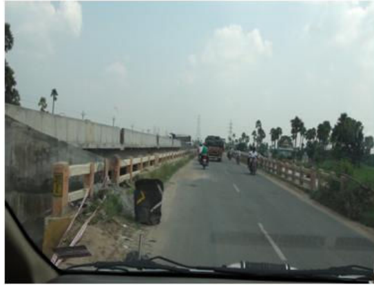
Fig.9: Cross drainage works without hazard markers a potential hazard during the night
