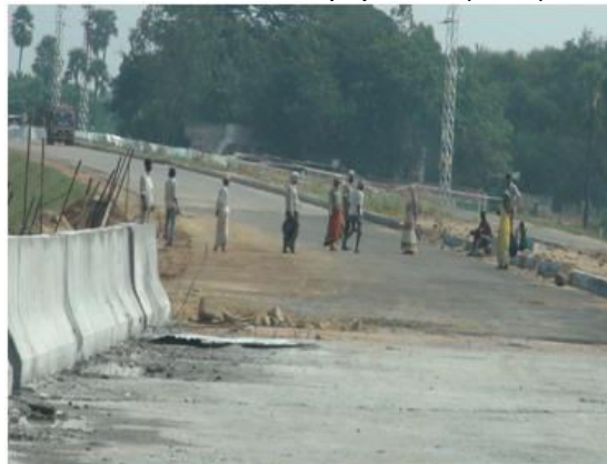
Fig.13: Workers are without any personnel protective equipment exposed to risk
