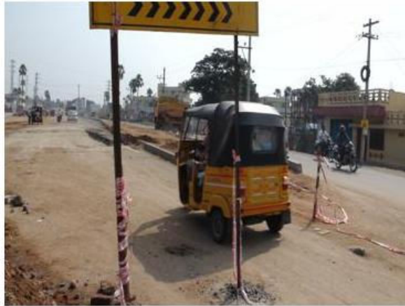
Fig 5: The traffic diversion was not properly made as result the all the traffic also passing through the construction zone resulting the potential accidents spots during the night time.
